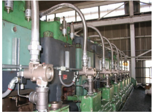
Cam actuated start valves with pressure-actuated in-head check valves
